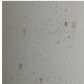
Water leaks = mold hazards
