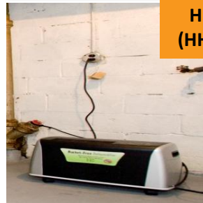
Remediate mold, install dehumidifier
