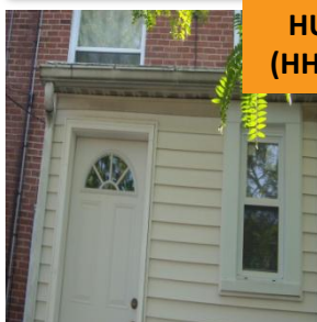
Replace broken gutters
