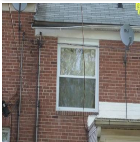
Defective gutters = water leaks
